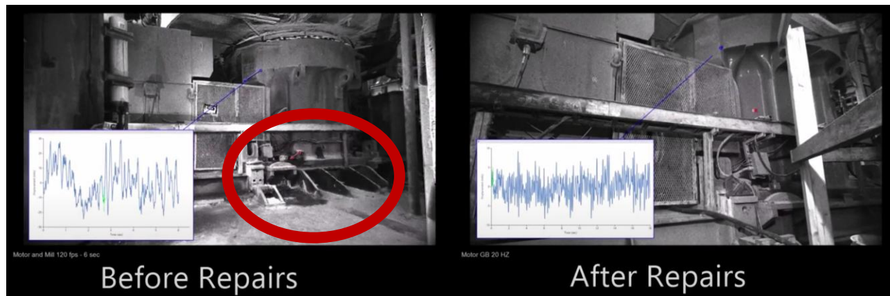
Fig. 1. Raw mill with significant base movement.
